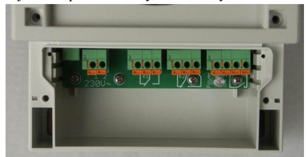
Electrical terminals of prh-ZG4
